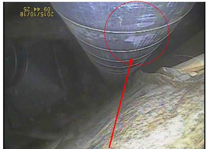
Signs of moisture damage on the outer wall of the chimney
