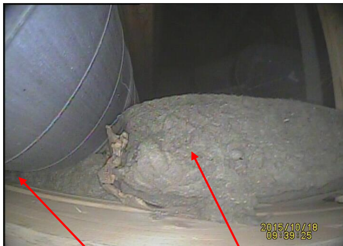
Inadequate clearance to combustible building materials and insulation, which are in direct contact with the chimney. This is a serious fire hazard
