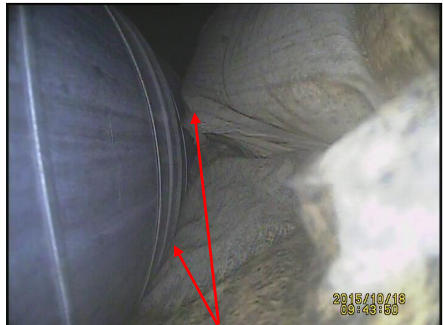
Combustible insulation in direct contact with the chimney. This is a serious fire hazard
