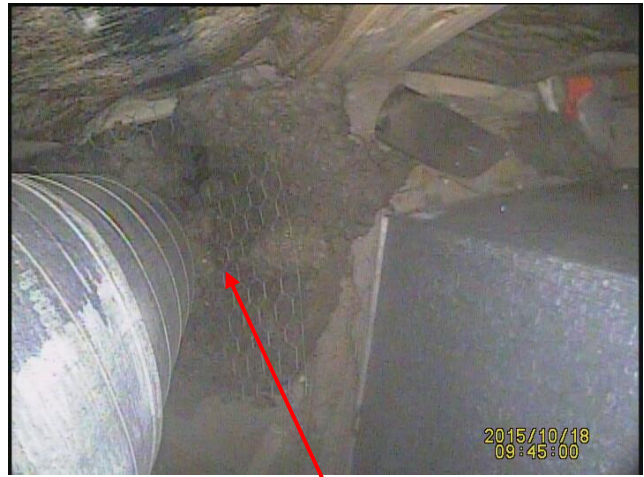
It appears that insulation has been placed on chicken wire in place of an adequate firestop. This is not approved and is a fire hazard
