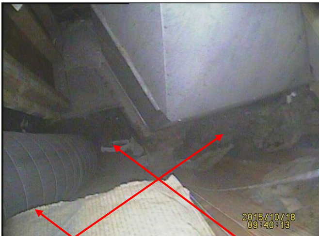
Insulation touching chimney & fireplace, a 2" airspace is required No firestop provided where chimney passes through floor/ceiling
