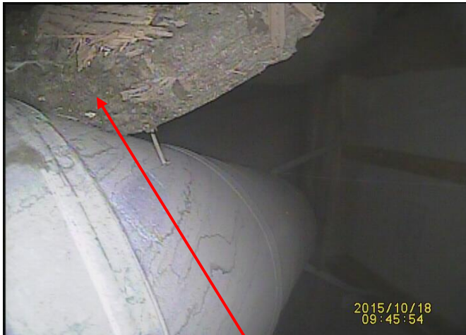
Combustible building material in direct contact with the chimney. This is a serious fire hazard
