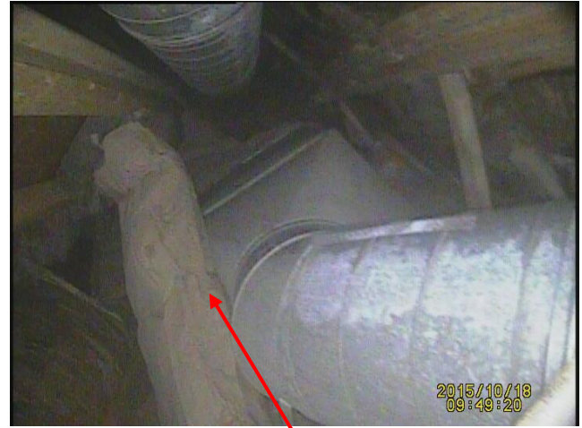
Insulation has fallen on top of a fireplace. This is a serious fire hazard
