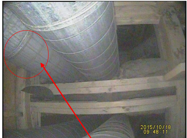
Lines of moisture running in and out of the seams of the outer wall of the chimney
