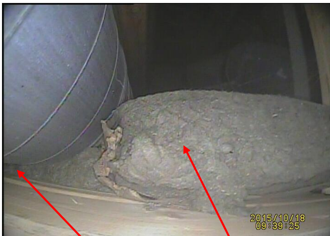
Inadequate clearance to combustible building materials and insulation, which are in direct contact with the chimney. This is a serious fire hazard
