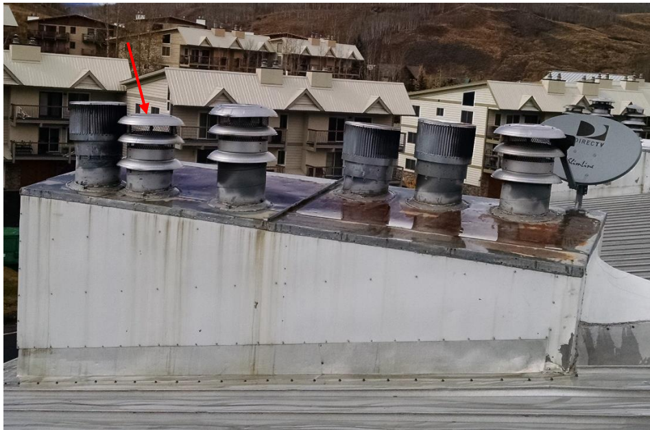
Manufactured Chimney System
