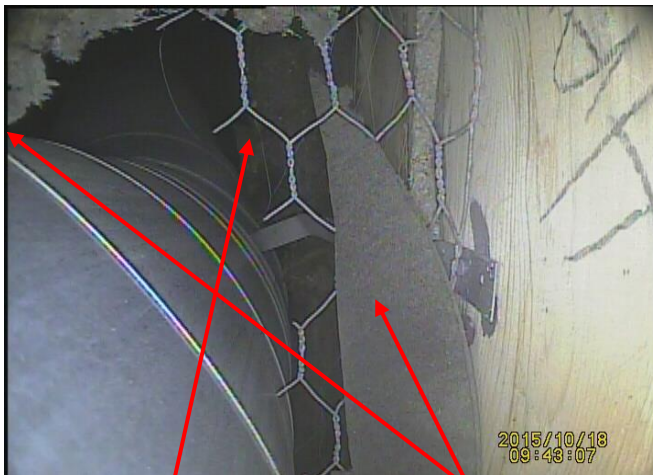
No firestop provided where chimney passes through floor/ceiling Debris touching chimney, a 2" airspace must be maintained
