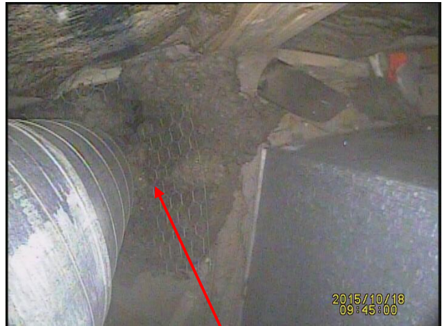
It appears that insulation has been placed on chicken wire in place of an adequate firestop. This is not approved and is a fire hazard
