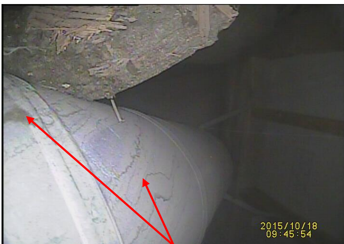
Signs of moisture presents on the outer wall of the chimney
