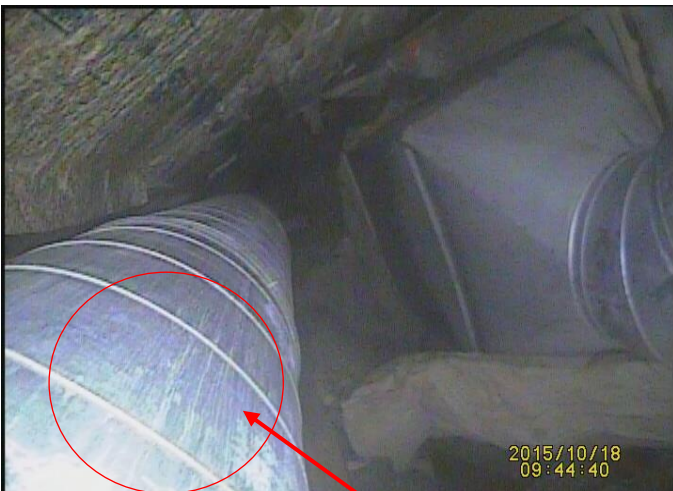
Lines of moisture running in and out of the seams of the outer wall of the chimney
