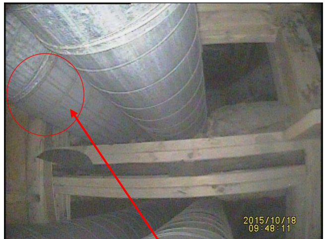
Lines of moisture running in and out of the seams of the outer wall of the chimney
